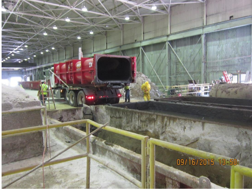
Crew emptying and cleaning out storage container contents into 40 ton half round.
