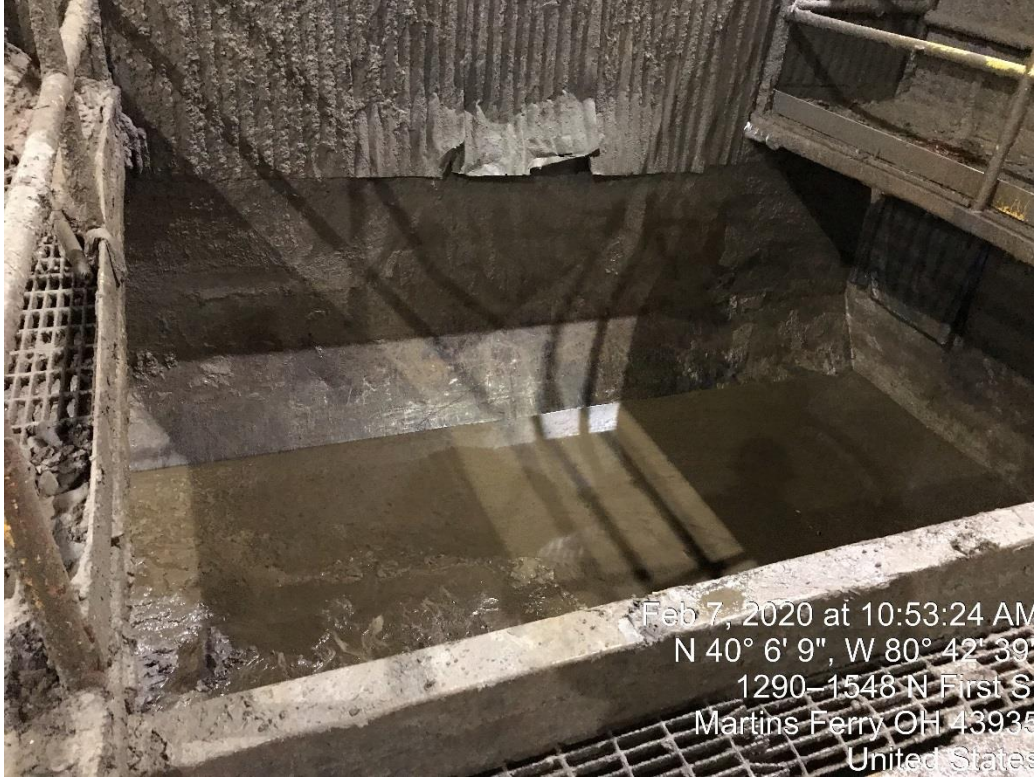
Low level TENORM mixing pit
