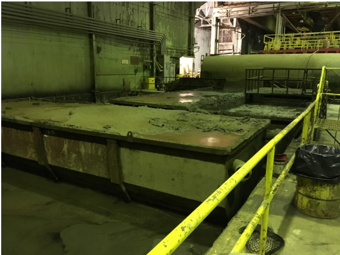
Overflowed halfrounds used to offload waste. Waste was observed inside the secondary containment pit.
