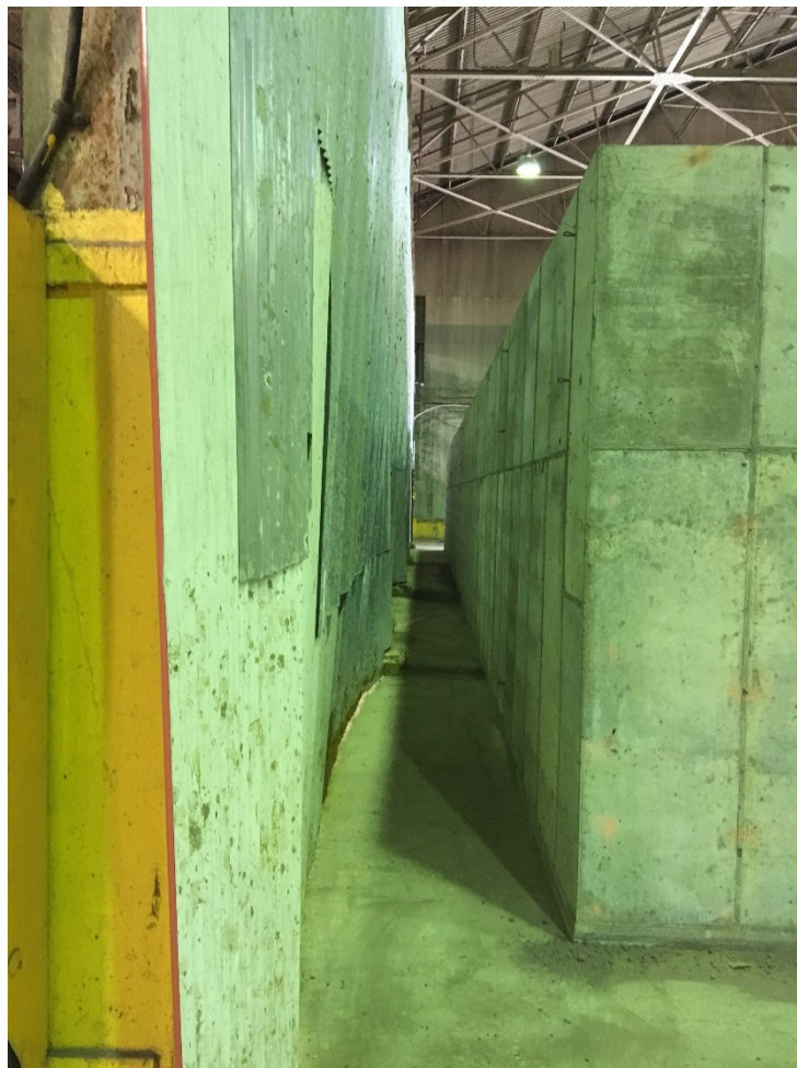
Improved housekeeping behind concrete bins
